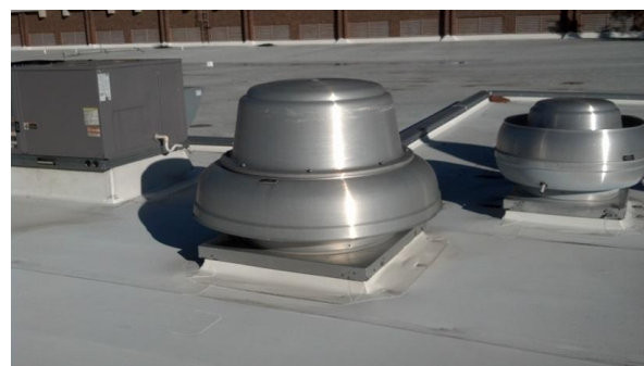
FIGURE 19. Typical Toilet Room Roof Exhaust Fan
