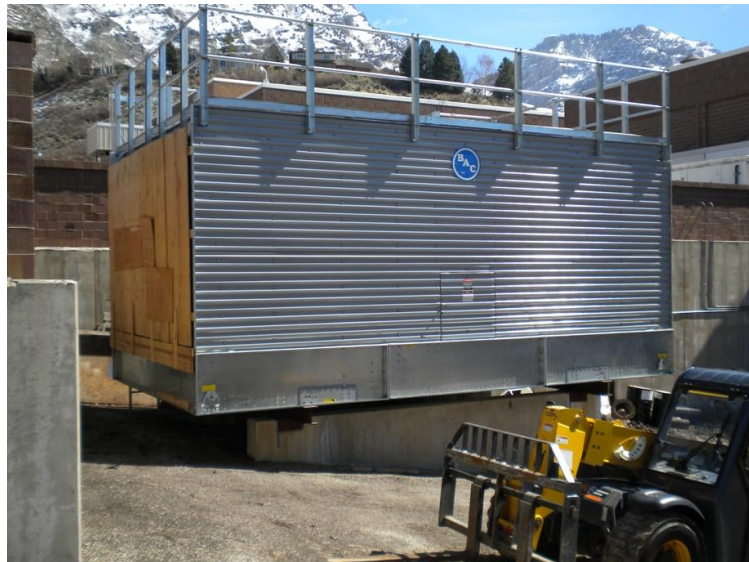
Figure 11. New Cooling Tower (2012)
