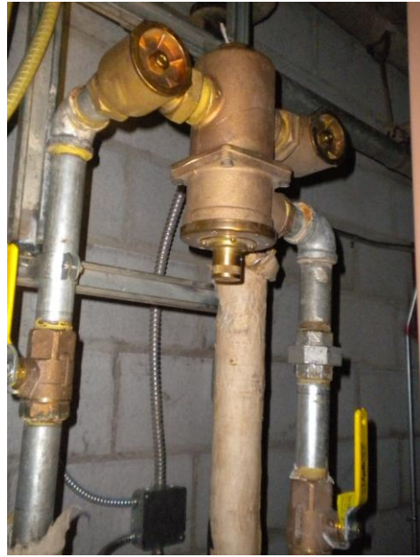
Figure 25. Galvanized Waters at Pipe Chase
