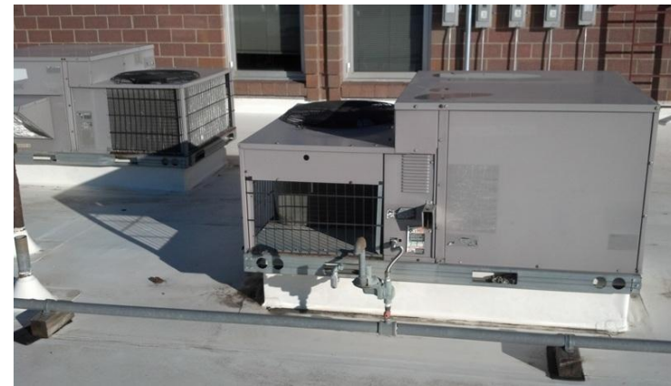
Figure 6. Typical Gas/DX RTU
