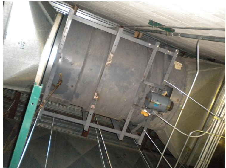
Figure 18. Return Fan Control in Mezzanine Fan Room
