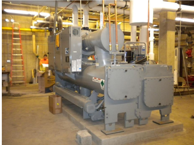
Figure 9. New Water Cooled Chiller (2012)
