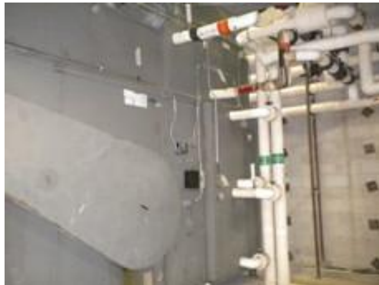
Figure 17. Existing Central Station Air Handler
