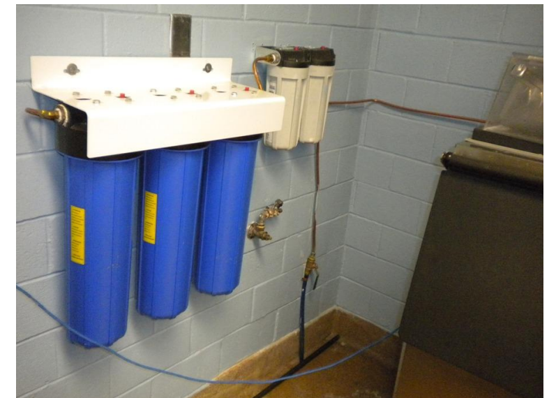
Figure 40. Kitchen Water Filters
