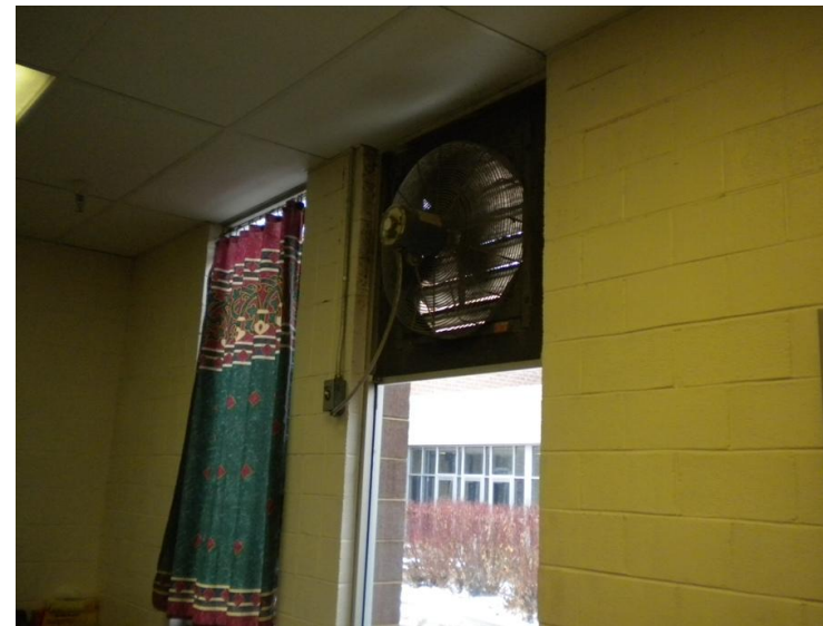
Figure 39. Prop Fan at Kitchen Dishwasher Area
