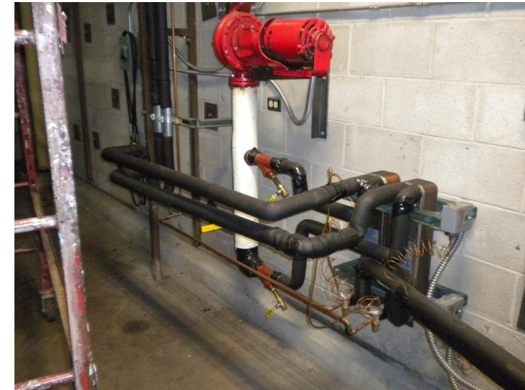
Figure 13. Administration Area Heat Exchanger
