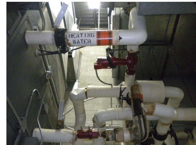
Figure 2. AHU Coil Piping & Coil Pump
