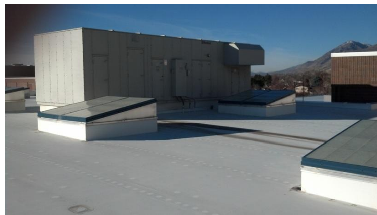
Figure 5. Gymnasium HW/CW Rooftop Unit
