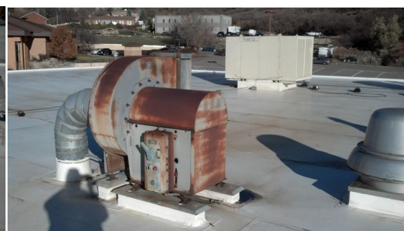
FIGURE 20. Shop Area Utility Exhaust Fan
