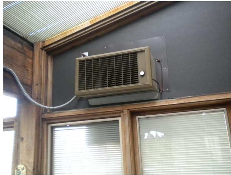
Figure 16. Greenhouse Evaporative Cooler
