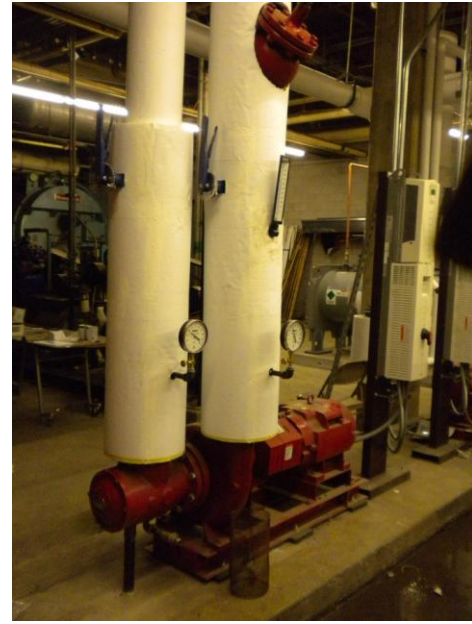
Figure 10. New Chilled Water Pumps (2012)
