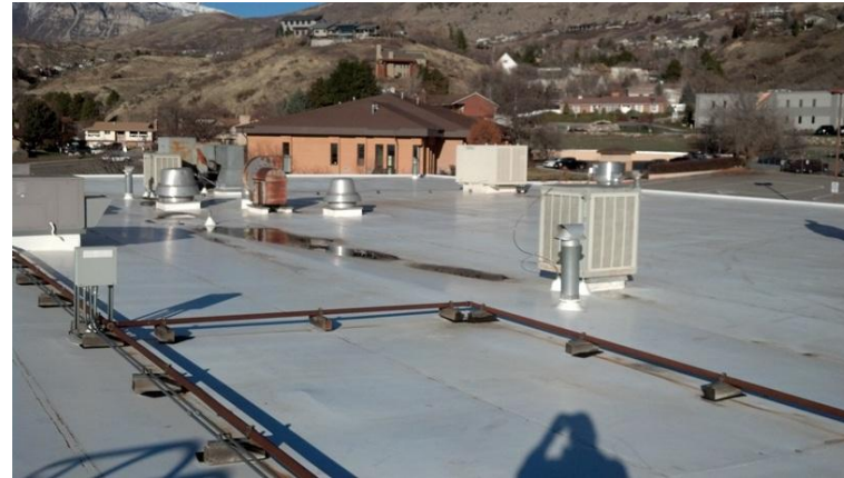
Figure 36. Typical Gas Piping Installation on Roof
