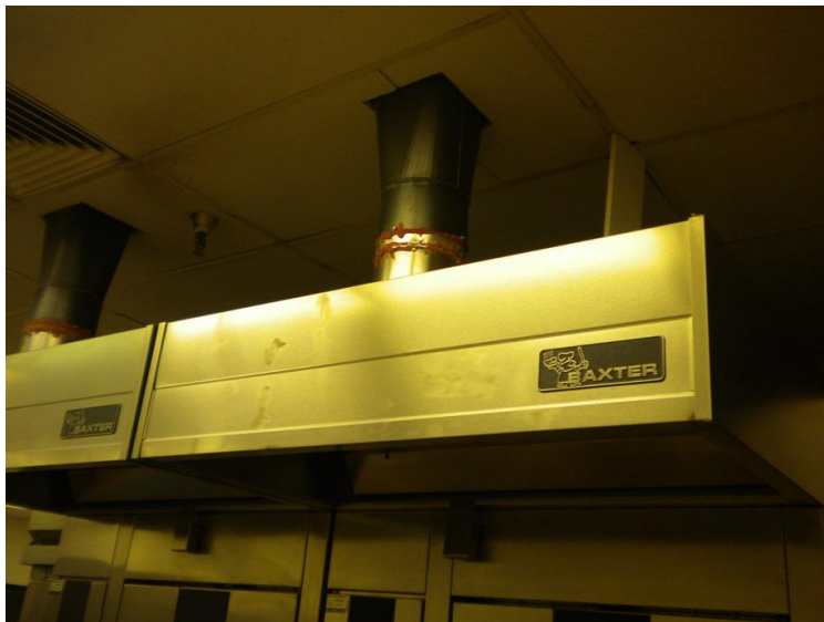
Figure 37. Kitchen Cook Hood
