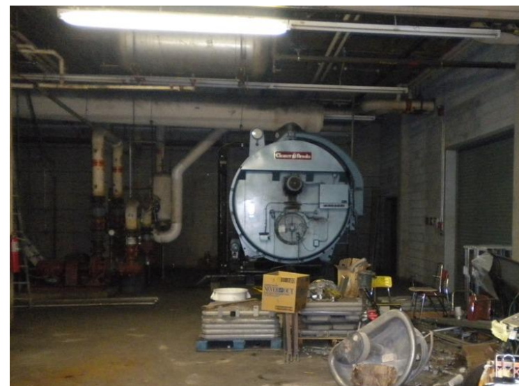
Figure 1. Existing Heating Boiler
