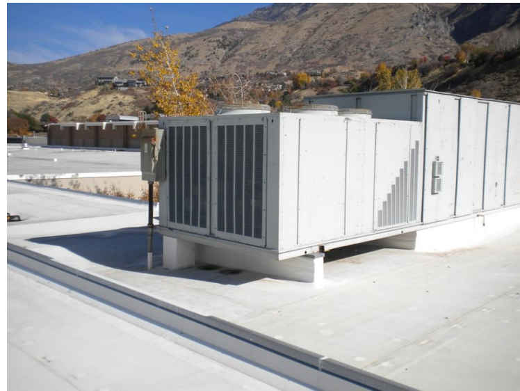
Figure 4. 1991 Classroom Addition Gas/DX RTU
