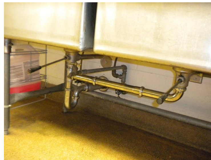
Figure 41. Hose Bibbs at Kitchen with No Vacuum Breaker Code Violation
