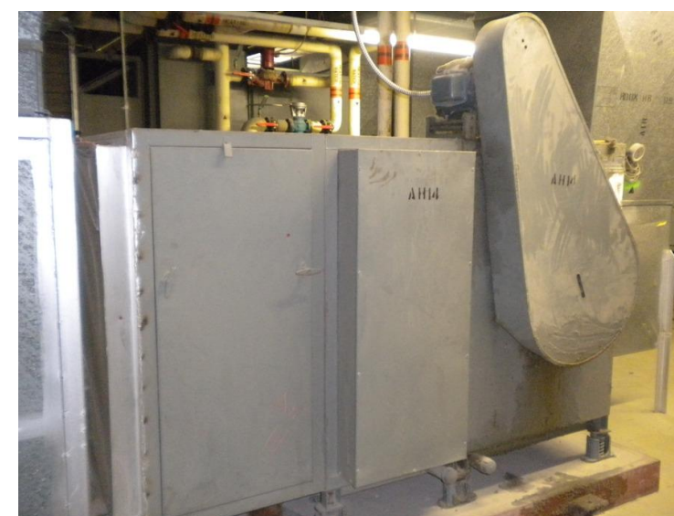
Figure 3. Existing HW/CW Control Station AHU
