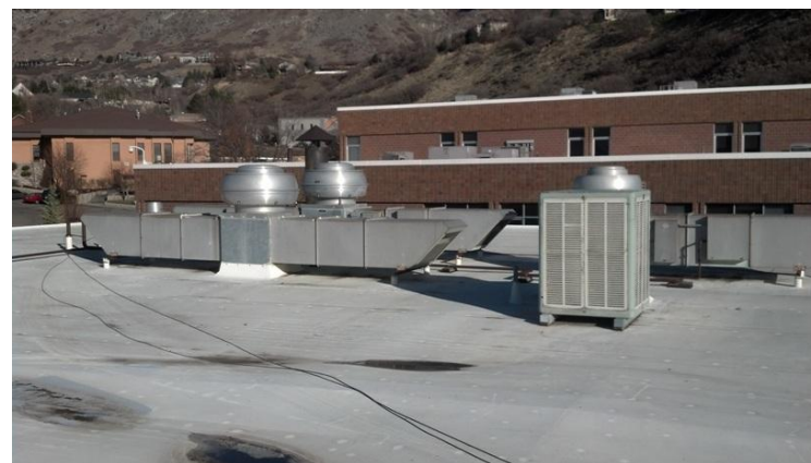
Figure 38. Kitchen Hood Make-Up Air/Exhaust System
