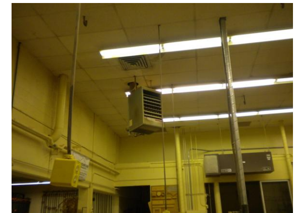
Figure 7. Shop Gas Unit Heater
