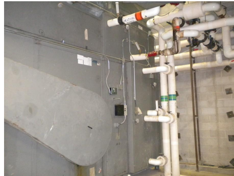
Figure 12. Existing Control Station Air Handler with CW Coil
