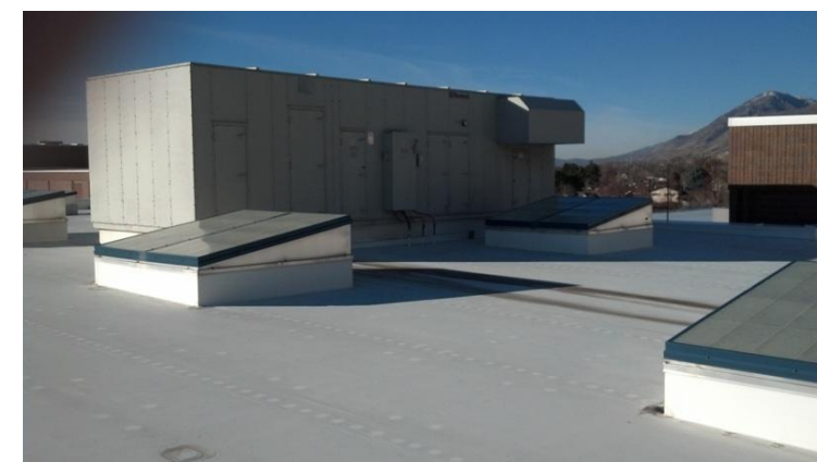
Figure 14. 1991 Addition Gas/DX Rooftop Unit
