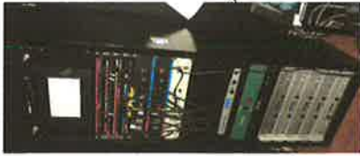
2 EXISTING AUDIO RACK IN LIGHT BOOTH
